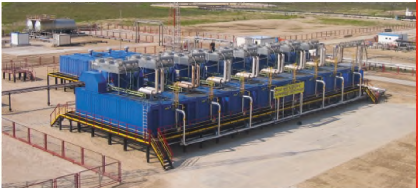
Bashneft Power Plant, Central Siberia
